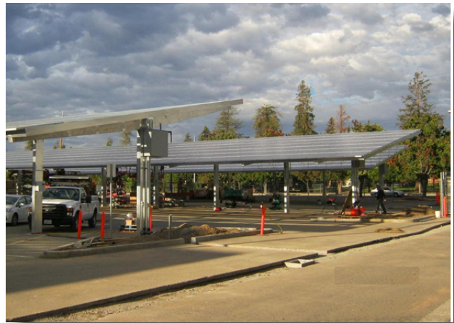
Solar-covered parking lot
