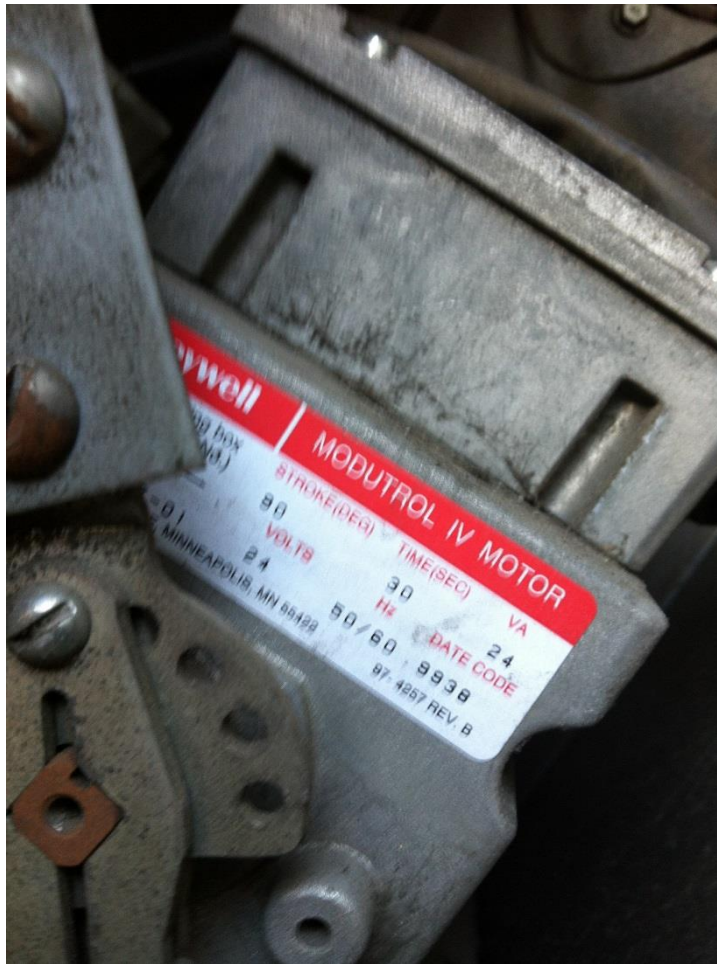
Figure 3.2: Broken Actuator Serving AC-1 OA and RA Damper set
