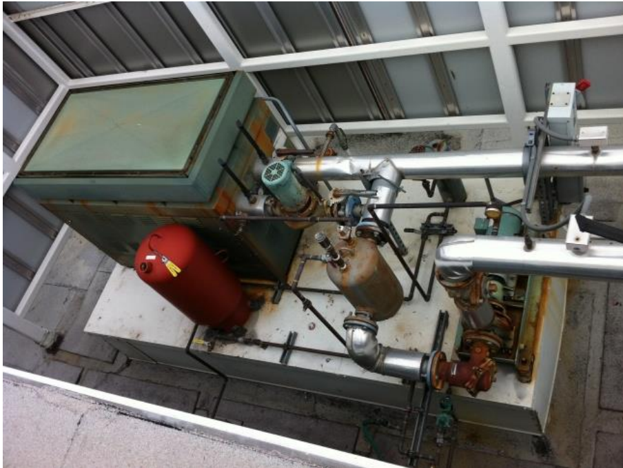
Figure 2.3: Boiler B-1, Providing HHW for the Civic Center
