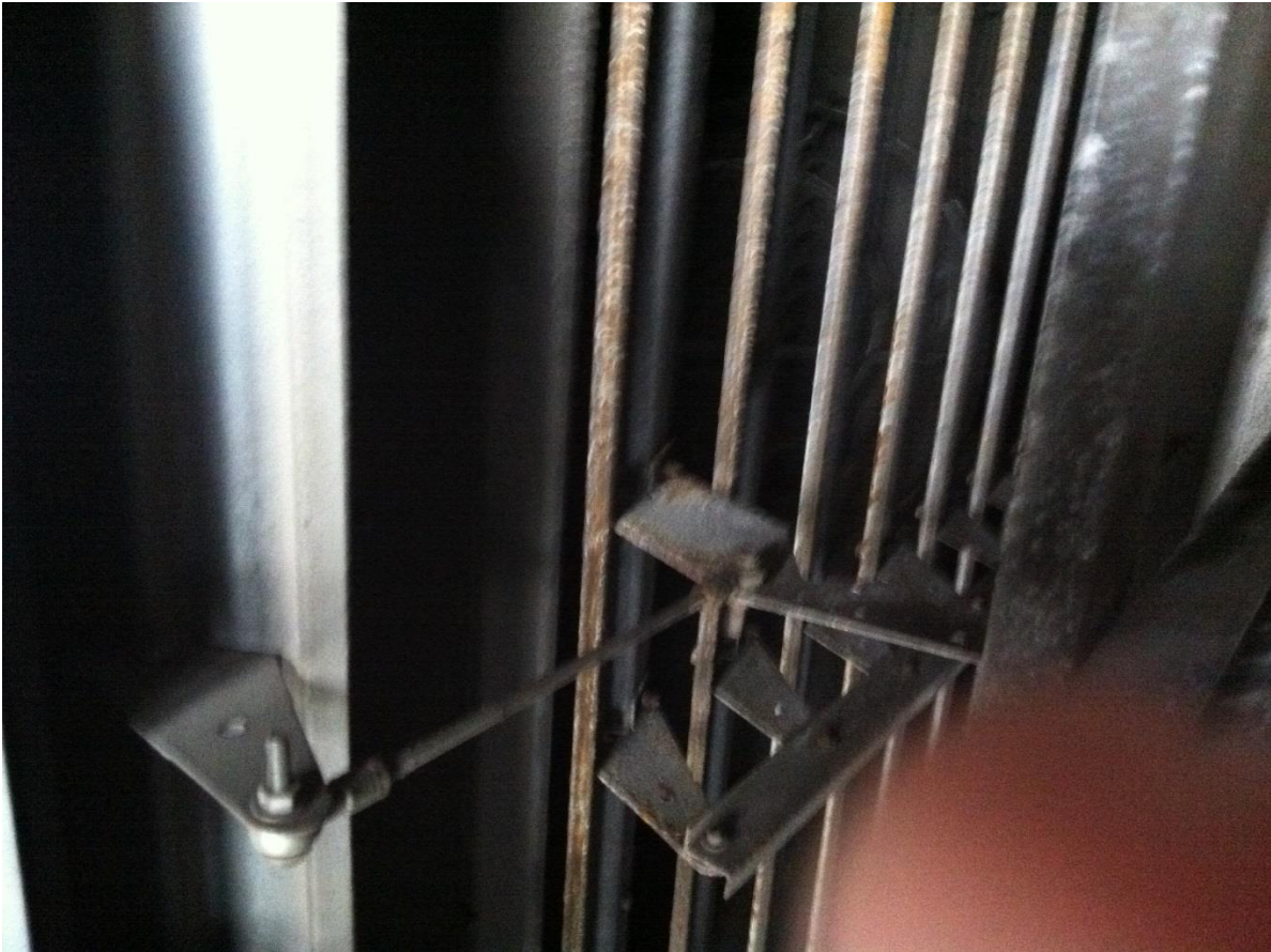
OA Damper set, Showing baseline linkage condition
