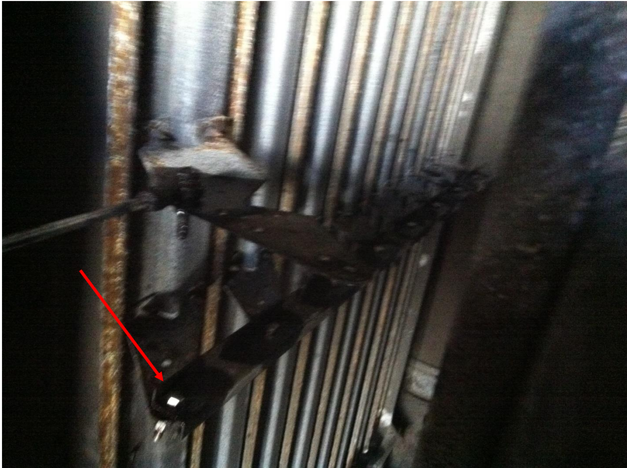
Figure 3.3: AC-1 OA Damper Linkage with new hardware
