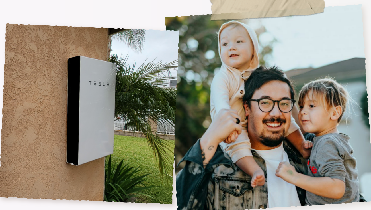
Tesla battery storage installed at a program participant's home (left) and community members enjoying the neighborhood (right)
