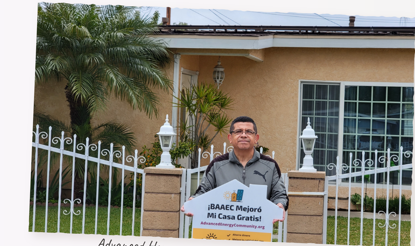
Advanced Homes program participant Juan Gonzalez on battery storage installation day at his home
