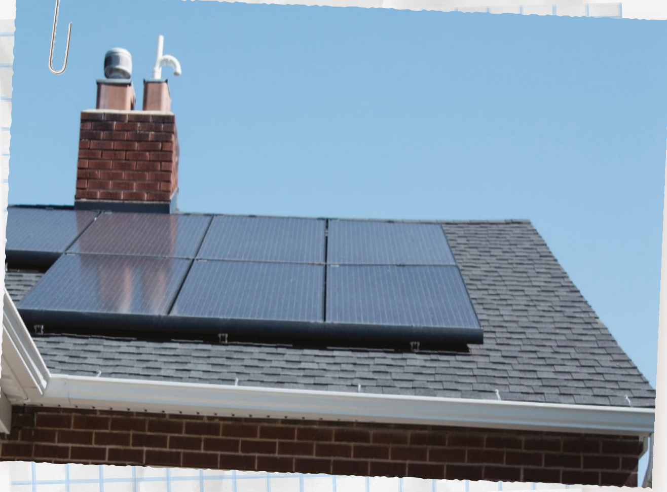
A Sunrun solar panel system installed by our project partner, GRID Alternatives
